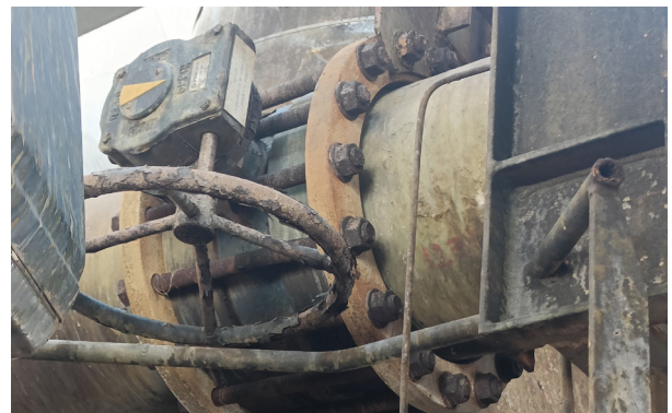
Figure 30. Example of a manual valve subjected to heavy corrosion by its environment and media.
