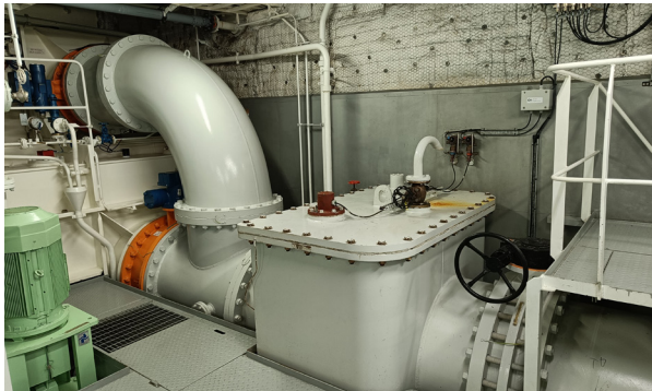
Figure 15. A sea chest filter with a manual inboard isolation valve on a passenger cruise ship. The valve outboard of the filter is remotely operated.
