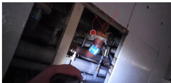
Figure 28. Engineer in the machinery spaces tracing the cooling system in search of a manual valve to be isolated as part of measuring the performance time for a simulated alarm response.
