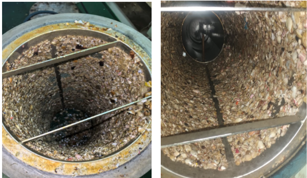
Figure 3.4 Low-temperature cooler filter No. 1 found with many bivalve shells captured on the filter mesh, when the filter was opened for cleaning on 17 th October 2024 (left picture) and again on 14 th April 2025 (right picture).
