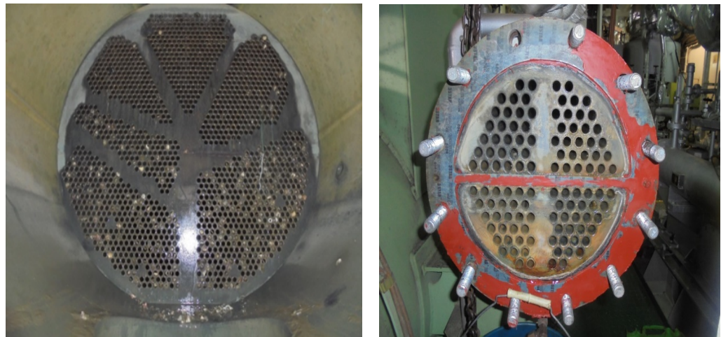
Figure 3.3 Vacuum condenser found on 30 th August 2024 with light bivalve shells blocking the tubes meeting fouling rating 3 (left picture). Air ejector condenser (right picture) found on 30 th August 2024 without marine growth, i.e., fouling rating 0.
