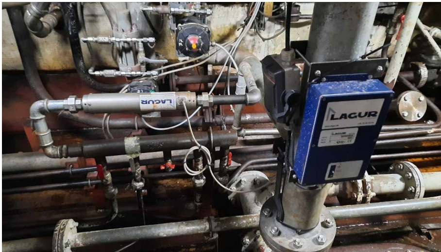
Figure 15.: Lagur system installed on ship engine fuel line before reaching the pre-injection mixer tank. The system was installed 6 months before the project began.
